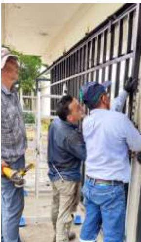
National and missionary workers repairing the entrance gate to our radio station's new home.
